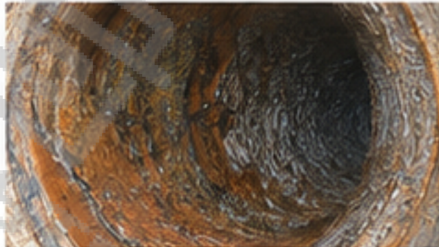
Typical CO 2 corrosion with FeCO 3 scale
